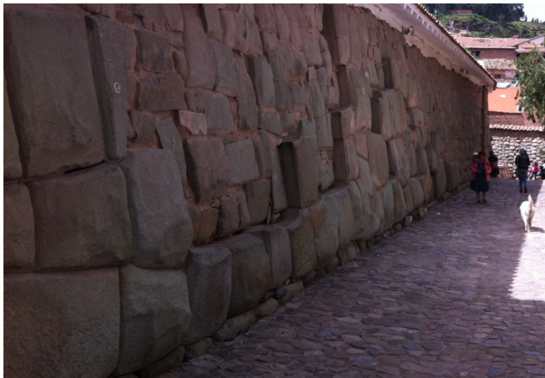
Figure 7: A earthquake proofing wall in Cusco, Peru. Note the small rocks at the bottom of the wall.
